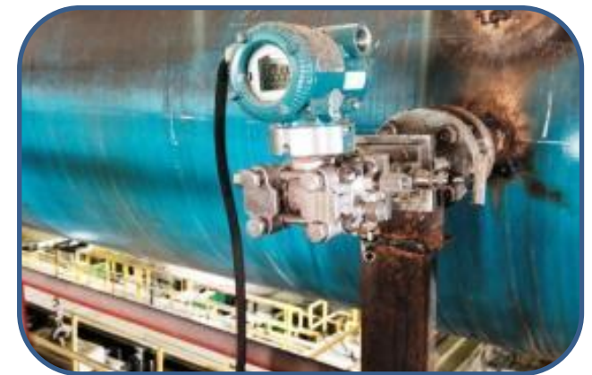
Flow Meter – Comb. Air Line
